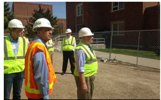
Petroleum Engineering Industry Advisory Council members tour the new Collaborative Energy Complex (CEC) building construction site.
